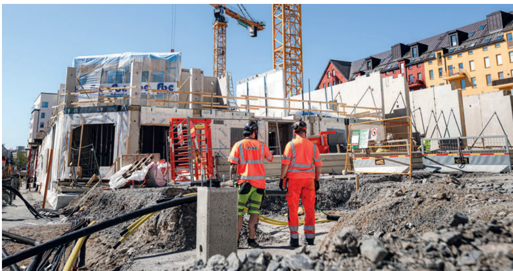
This residential project Persikan in Södermalm is currently being built with precast elements from the new factory in Hallstahammar.
