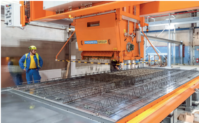
The eCon Drive concrete spreader in the factory in Ucklum can produce 5 pallets per hour with 28 m 2 per pallet.
